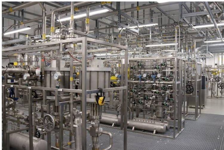
Fig. 6: View of P5.2 gaseous panel room
