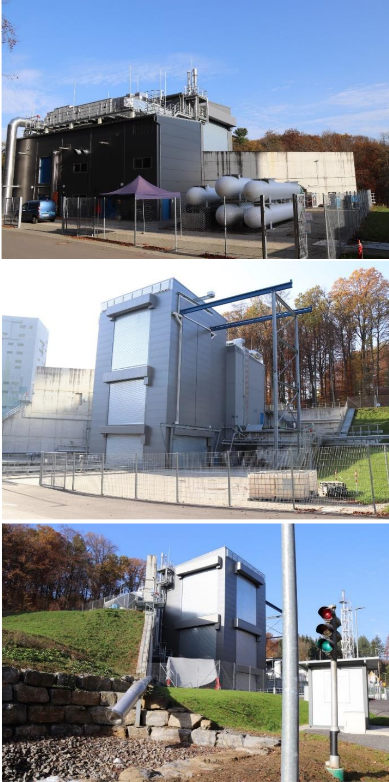
Fig. 5: Test bench P5.2 from different angles: high-pressure bottles and concrete building (top), chute area and crane device (middle), LOX basin and flare stack (bottom)
