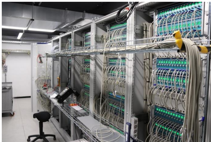
Fig. 8: View of P5.2 front end room of P5.2 MCC
