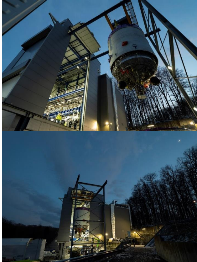
Fig. 11: ULPM integration into P5.2 test facility (© ESA)
