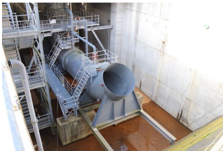
Fig. 7: View of P5.2 exhaust jet guiding system
