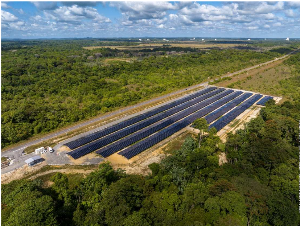
Photo 2 : Drone photo of CPV2 photovoltaic field (FR2030)
