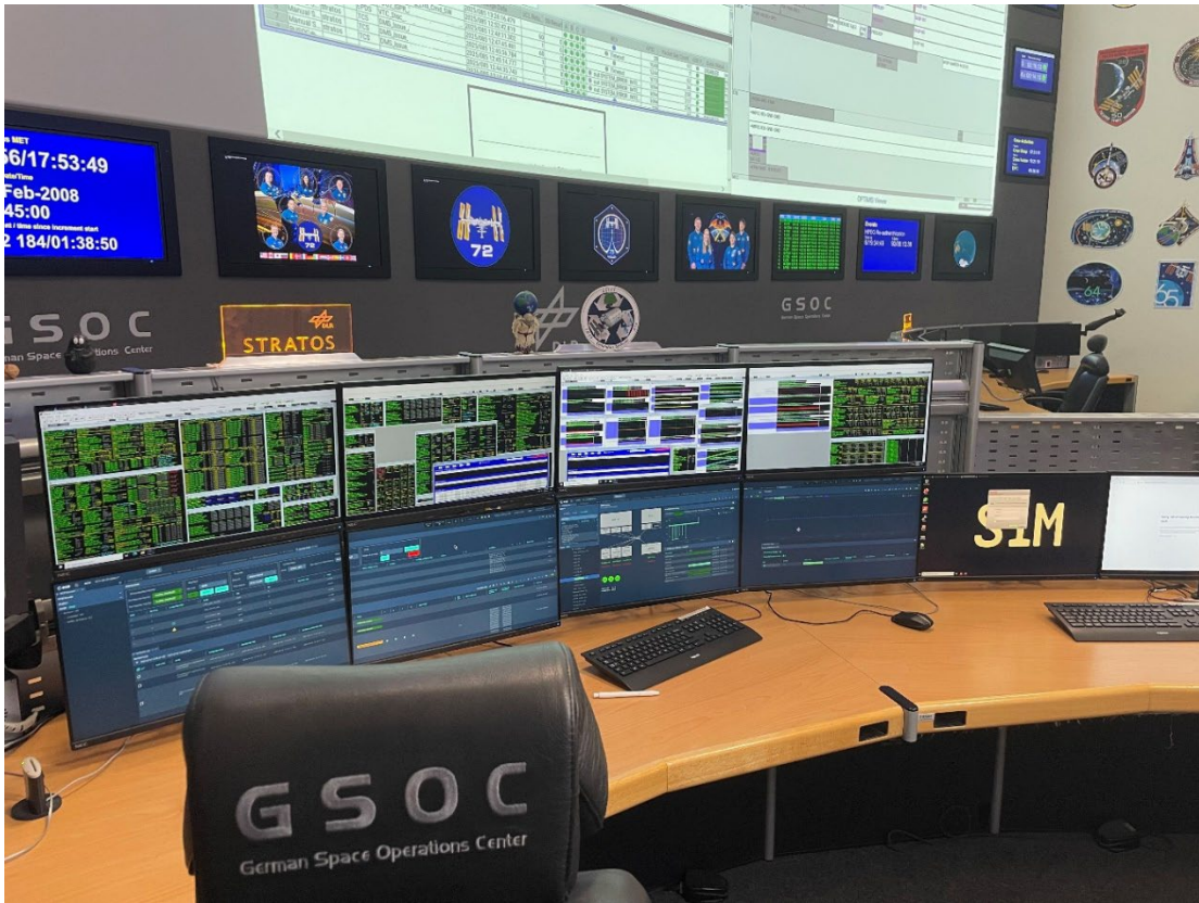
Figure 8 A view of the STRATOS console in one of HECC's control rooms with the new MCS-R clients running on the lower screens
